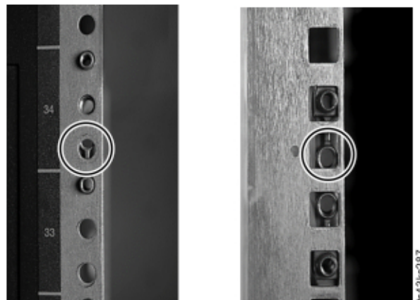
Figure 30. Incorrect connector locations
